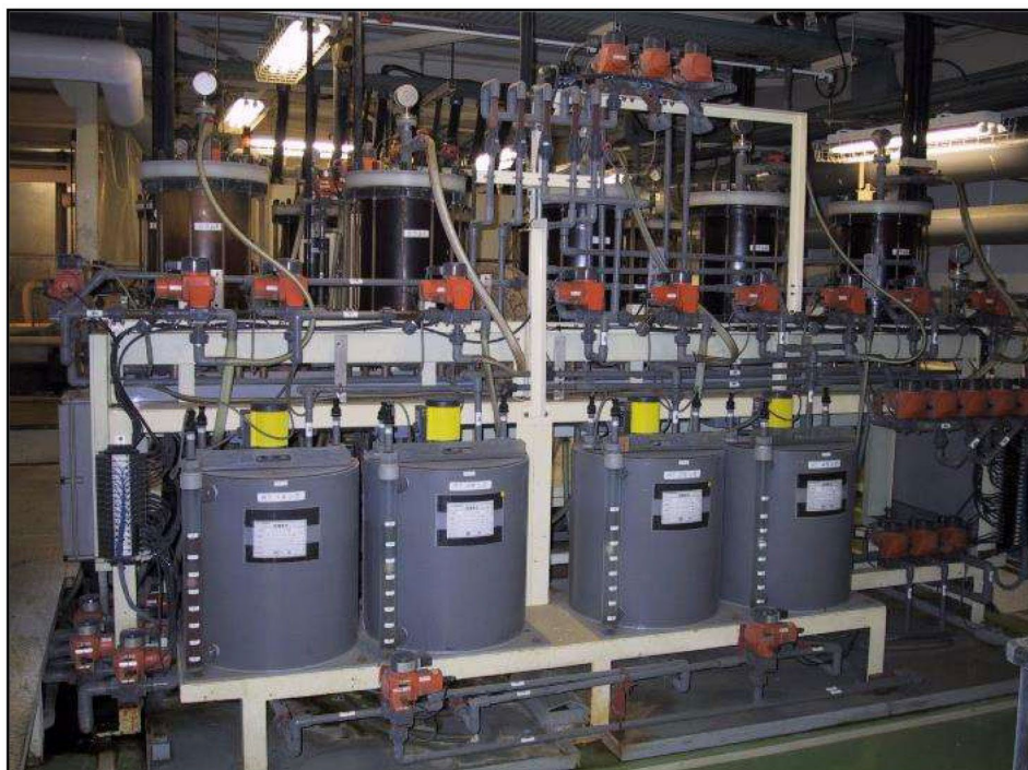
Figure 8. MRT™ Industrial Facility for Rhodium Separation and Recovery at Tanaka Kikinzoku Kogyo K.K. Reproduced with permission from [2].
